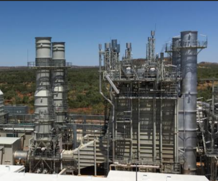
Diamantina Power Station in Qld
