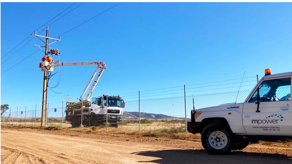
Image: Grid connection of the 5MWac solar farm at South Hummocks, South Australia
