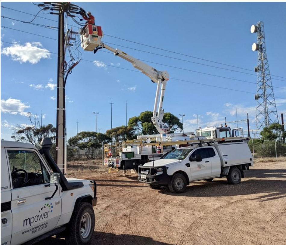
Image: Grid connection of the 5MWac solar farm at Kadina, South Australia
