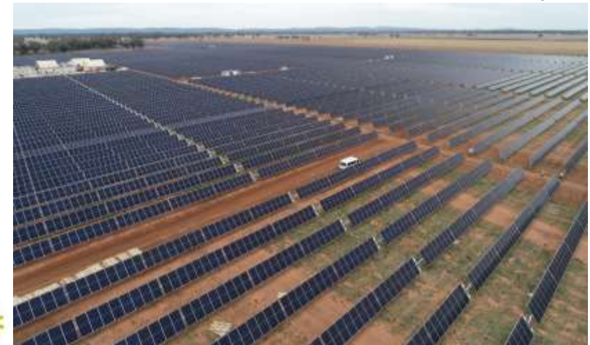
Jemalong 50MW Solar Project
