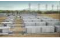
50MW Bouldercombe Battery
