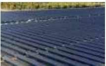
50MW Jemalong Solar
