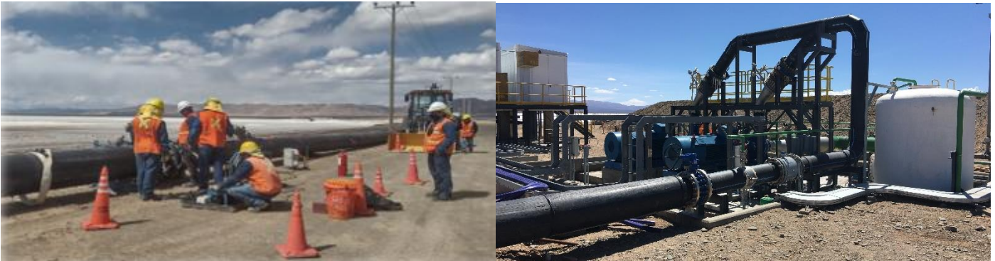
Note: brine gathering network under construction and gathering pond TK1100 pumping station
