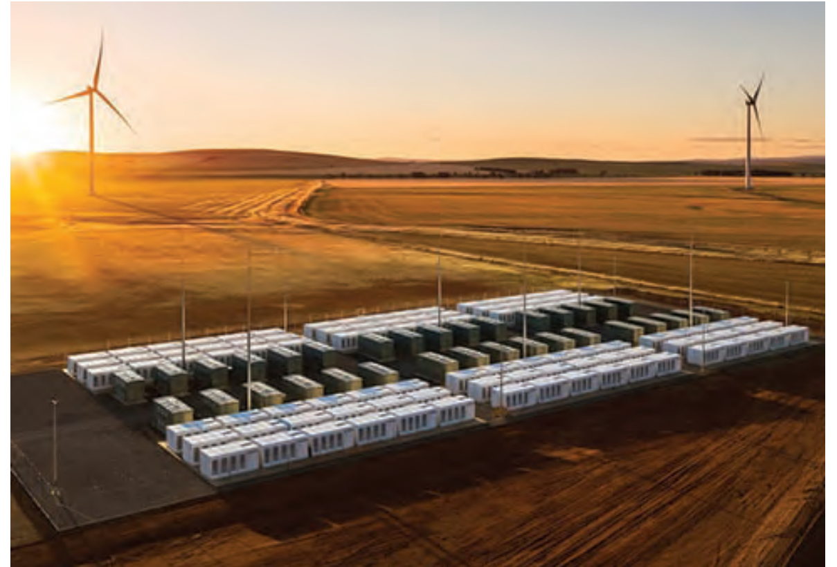
Tesla 100-MW/129-MWh energy storage system, Hornsdale Wind Farm in South Australia . Courtesy: Tesla
