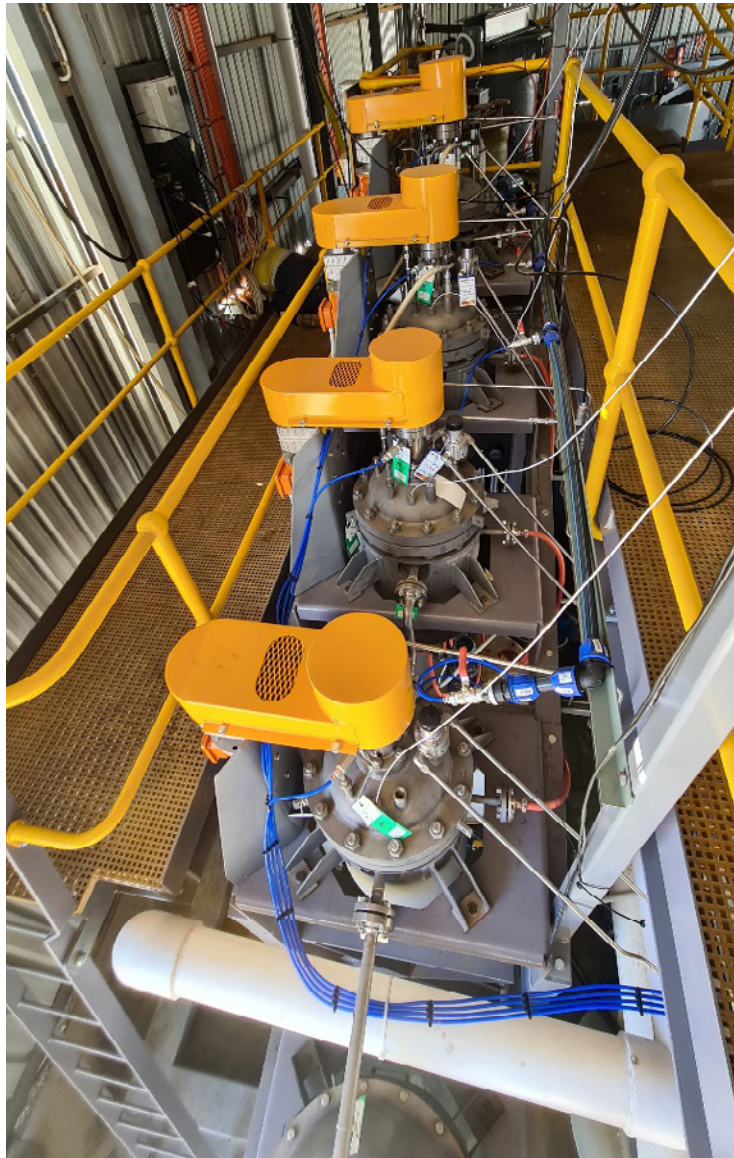
Figure 2 – Broken Hill Cobalt Project – Pressure Oxidation Circuit
