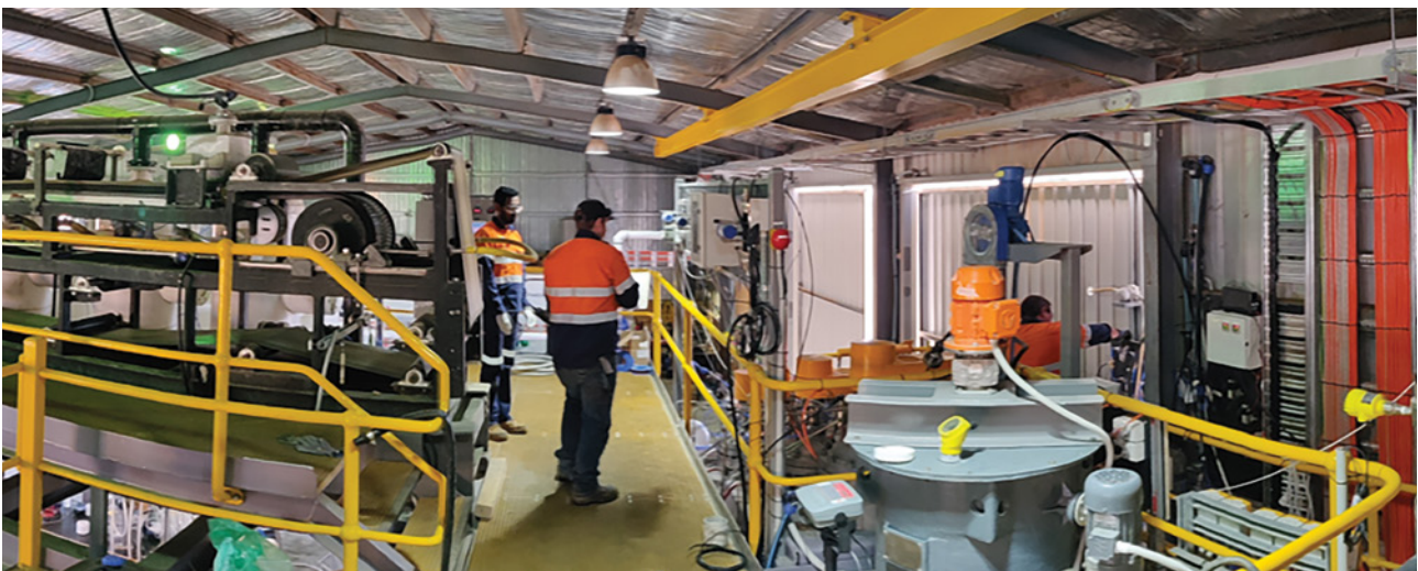
Figure 3 – Broken Hill Cobalt Project – Belt Filter & Pressure Oxidation Circuit
