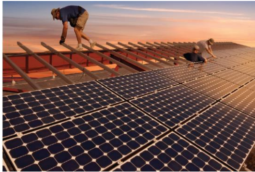
Solar panels, construction and commercial
