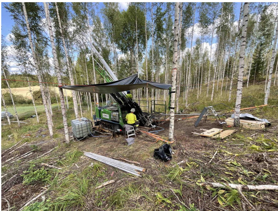
Figure 2: Taratest Oy GM85 drill rig operating on drillhole SM0008. Small track mounted rig for low environmental impact.
