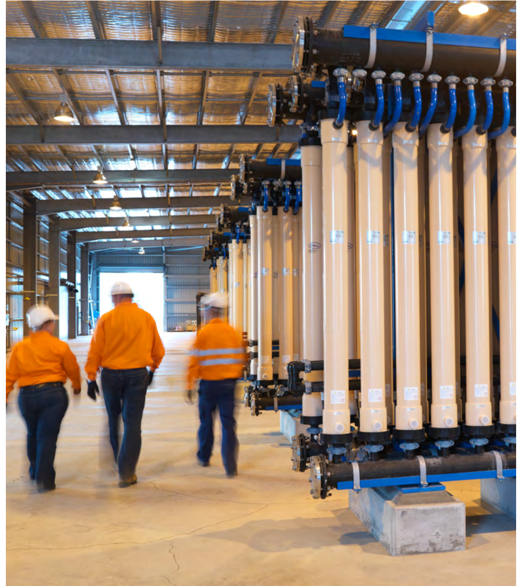
▲ The Talinga Water Treatment Facility uses reverse osmosis to prepare water for beneficial uses such as crop irrigation.
