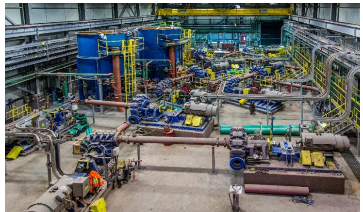
New tailings pumping system
