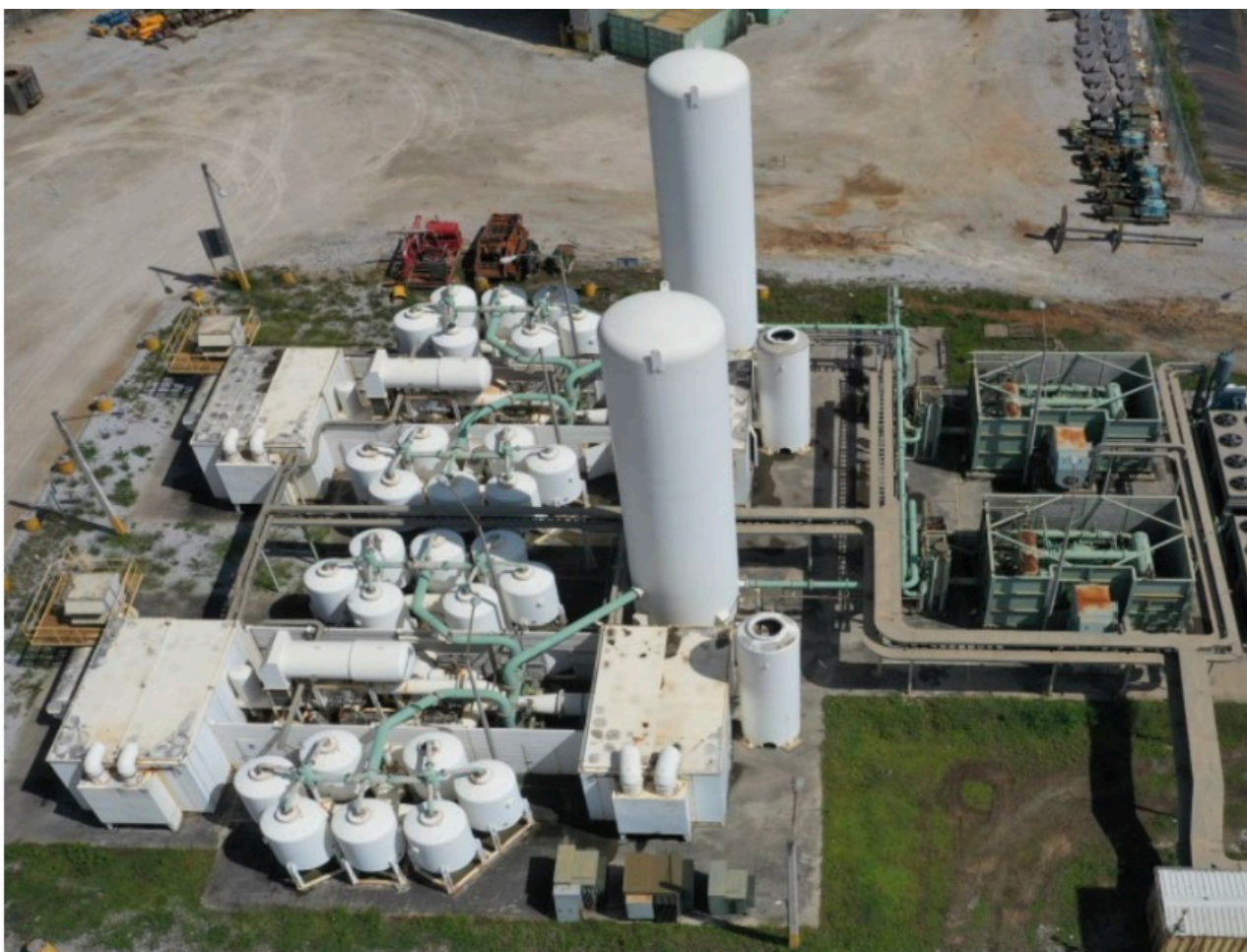
Antilles Gold's Oxygen Plant for potential use in a new concentrate processing facility
