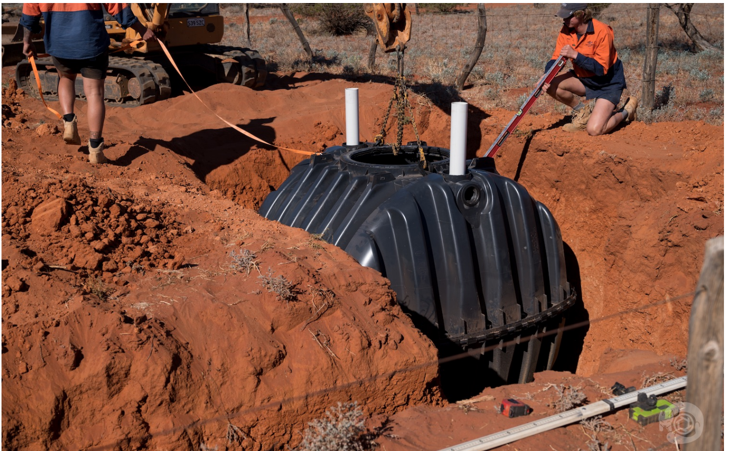
Figure 11: Septic tank facilities being installed, much to the delight of the team (May 2021)
