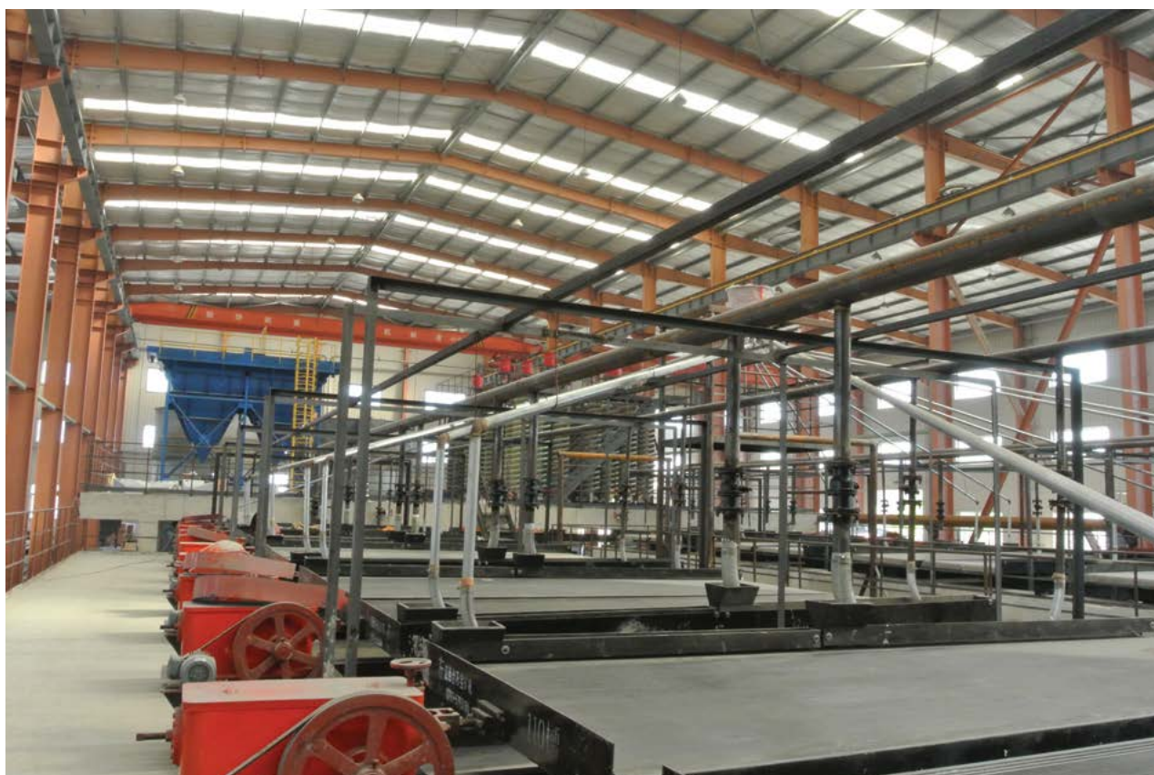
Shaking tables, Astron's Yingkou mineral separation plant, China and storage bins below.
