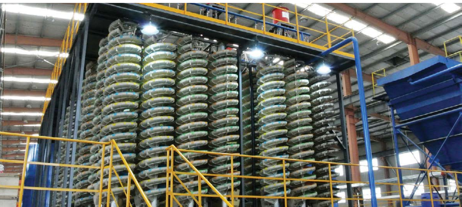
Spiral banks at Astron's Yingkou mineral separation plant, China.
