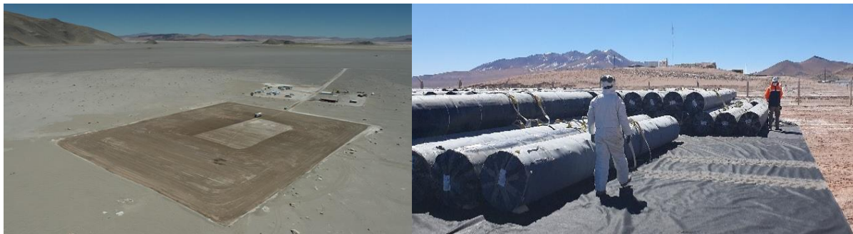
Figure 1: Sal de Vida – laydown area of construction camp (left) and arrival of pond liners to site (right)
