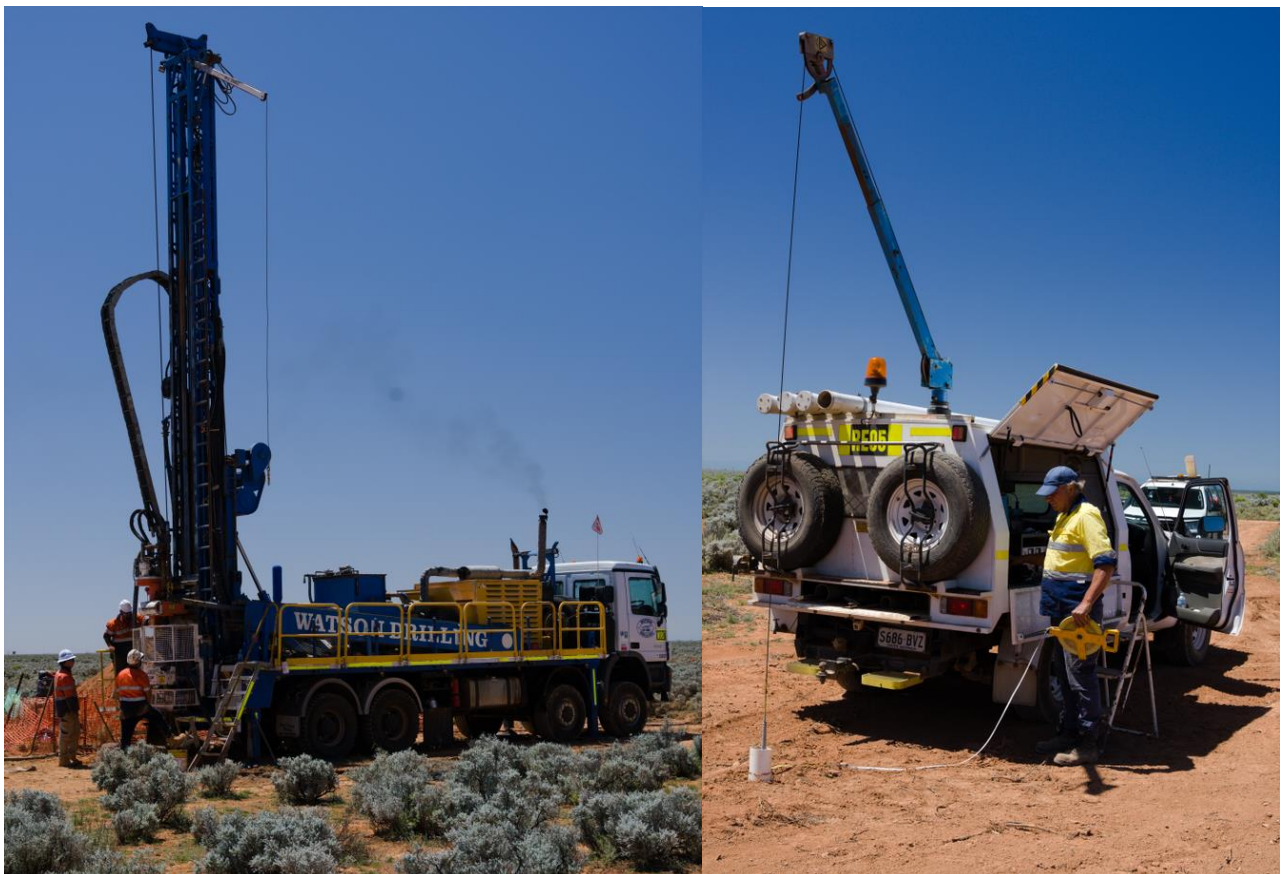
Figure 2: Rotary mud drilling rig and down hole logging onsite at Blackbush deposit, Sapphire Uranium Project
