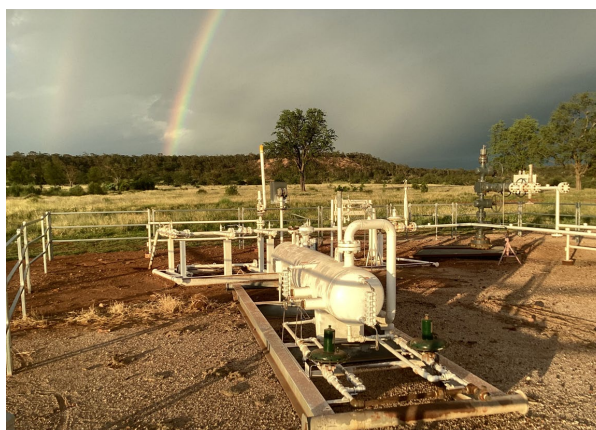
Warroon #1 – Well Head Facilities & Separator
