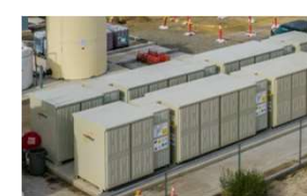
2 MWh system implemented in US
