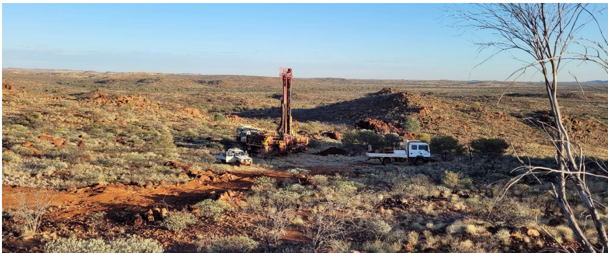
Figure 1: RC drill rig collaring the first hole into the gossanous horizon along the Money Intrusion at Mangaroon.
