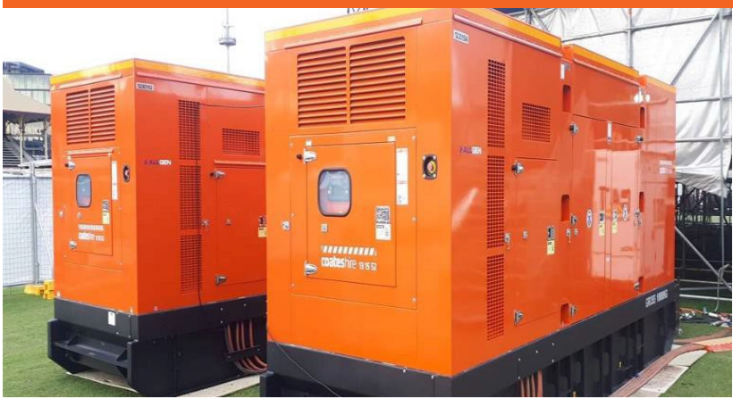
Power and HVAC Solutions
