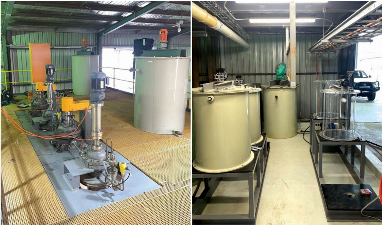
Figure 6 – Broken Hill plant. Left: Iron oxidation and precipitation circuit. Right: Installation of iron polishing and MHP precipitation circuits.
