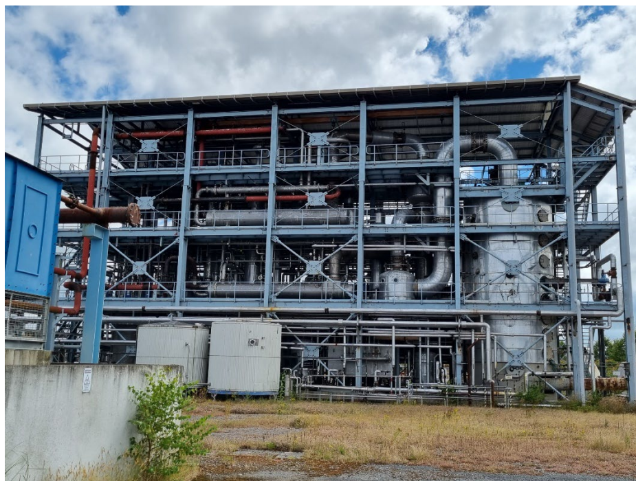
Leaf's upgraded plant equipment in New Zealand
