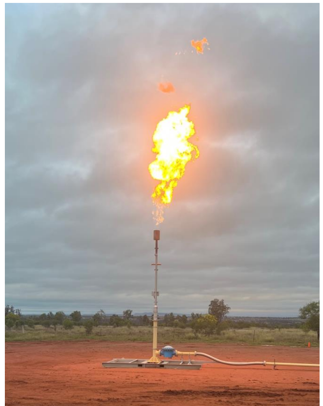
Figure 3 – Mahalo North 1 flare
