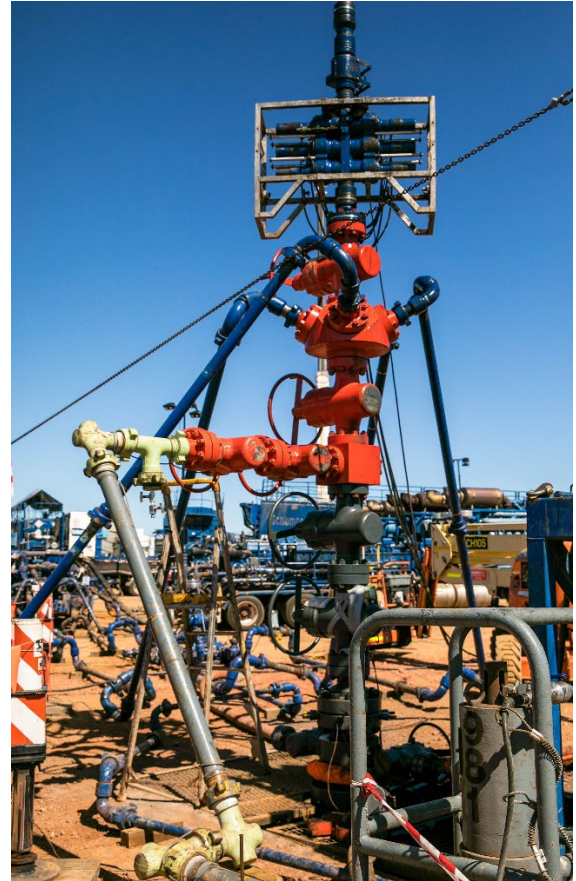
Carpentaria-2H high-pressure hydraulic stimulation wellhead
