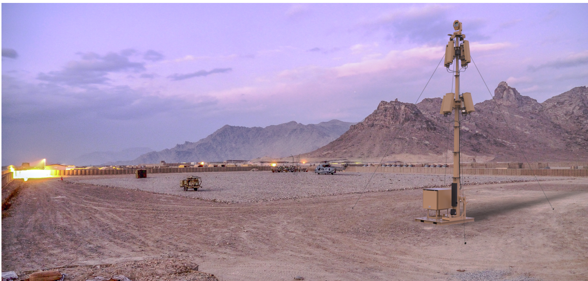
Image: DroneShield DroneSentry® system including RfOne® detection sensors and DroneCannon® defeat devices
