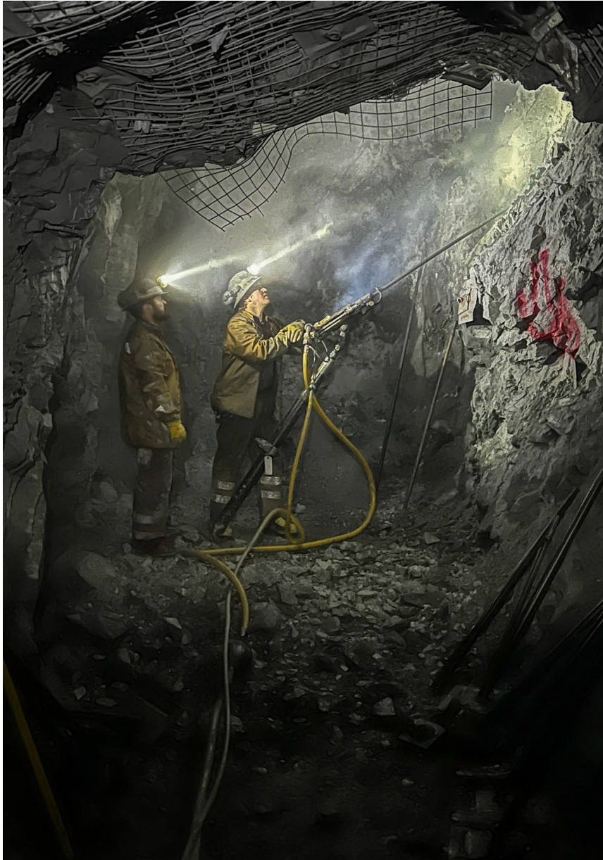
Figure 4 Handheld mining on high grade 2150 vein at the Morris Winze area minimises dilution of the ore zone
