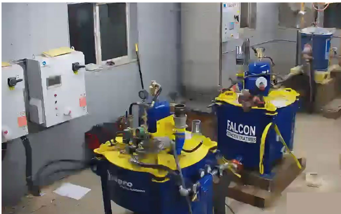
Figure 8 Falcon Concentrators being craned in, worked on and in place at the Lucky Strike Mill facility
