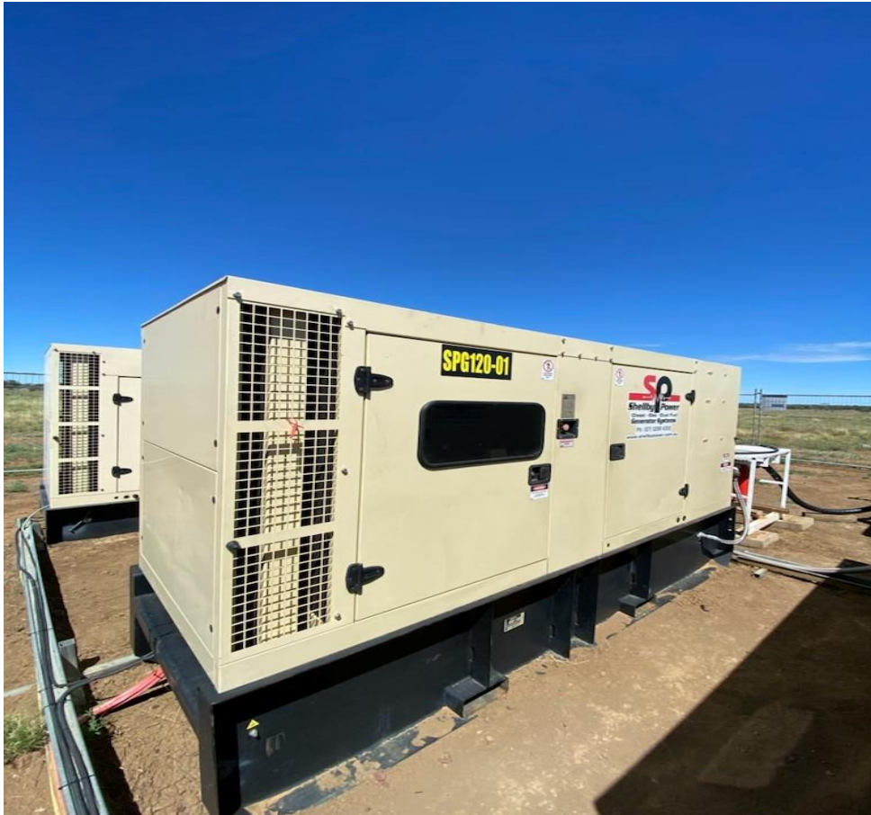
Gas-only generator installed at site
