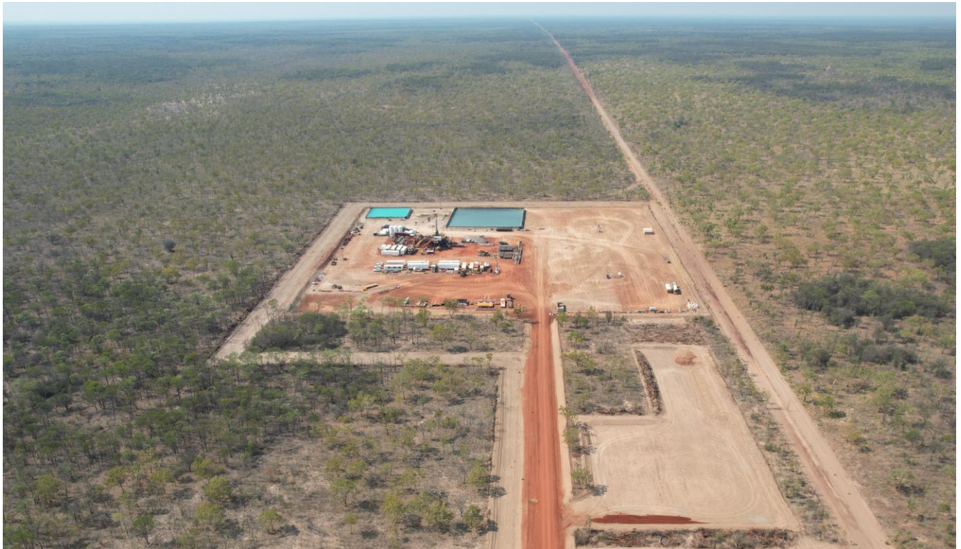
Figure 2: Well pad and preparation for the drilling of Amungee 2H in EP 98
