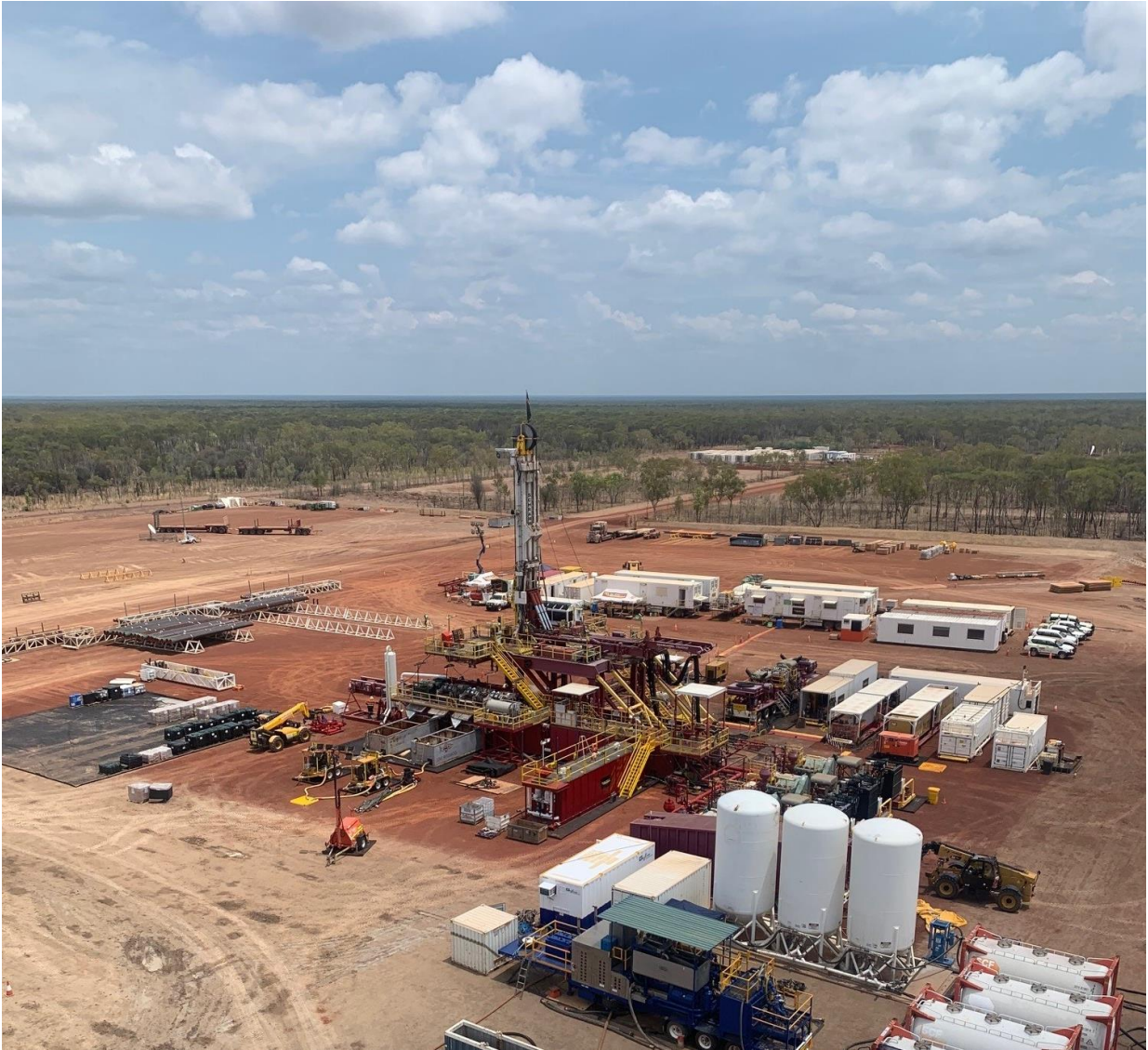
Figure 2: Well pad and preparation for the drilling of Amungee 2H within EP 98
