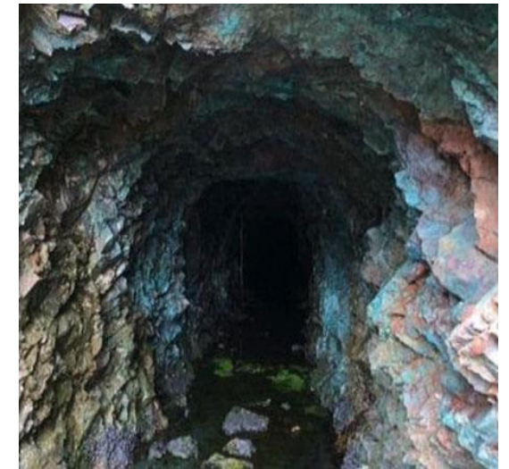
Tunnel at Andrade ridge. The photo was taken by the team in 2019.
