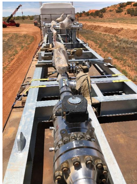
Delivery of manifold skids to Vali site
