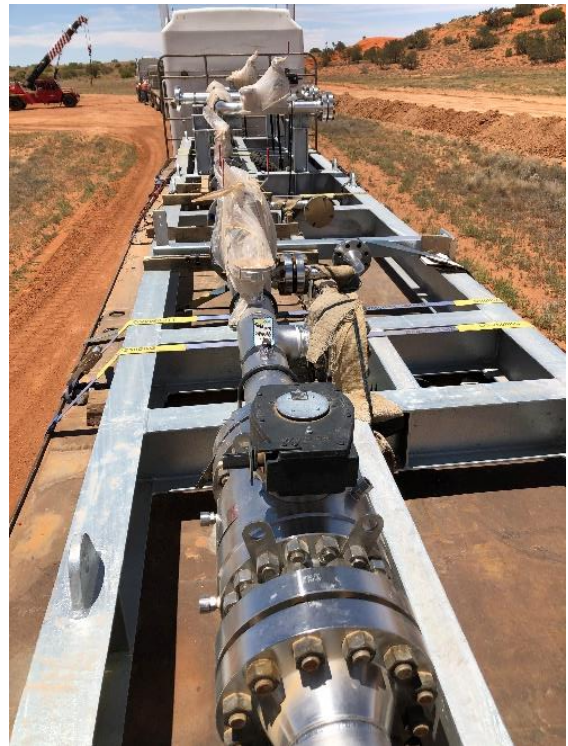
Delivery of manifold skids to Vali site
