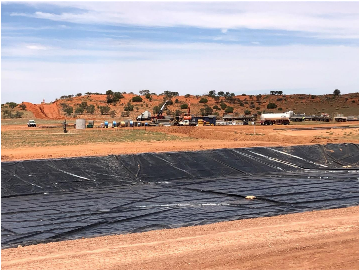
Installed pond liner with Vali-1 well site and laydown area in the background
