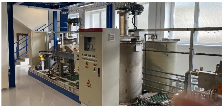
7. HPMM Dissolution, Deep Final Purification Module
