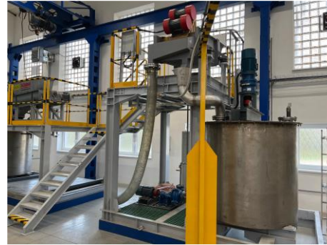
1. Ore to Slurry Preparation Module
