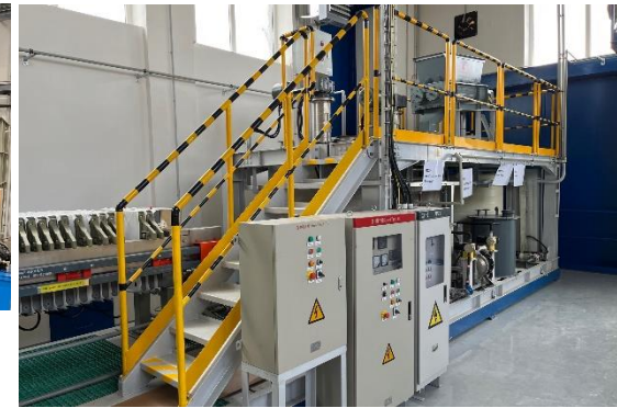
4. Leaching and Purification Module
