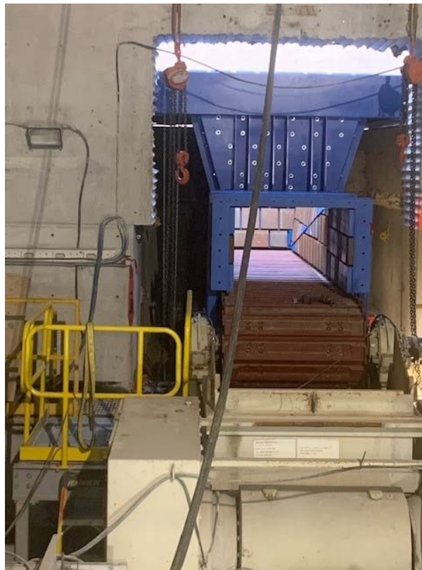
Figure 3: Apron Feeder and chute
