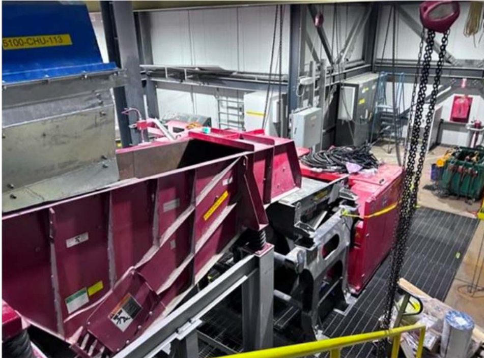
3 rd Ore Sorter mechanical and electrical installation
