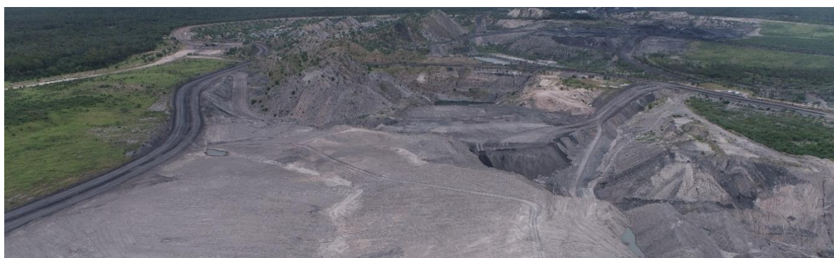
Image 1 - Completed northern end of Stage 1 (FY23) rehabilitation. The dumped out West Pit ramp can be seen at the northern extent of the dozer push.
