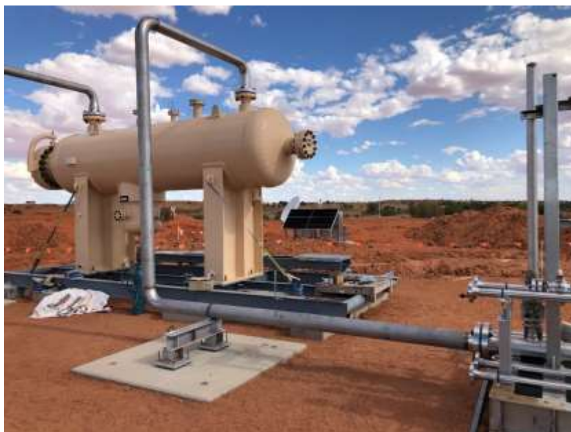
Separator installed at the Vali metering lease
