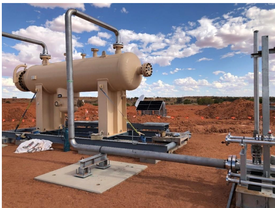
Separator installed at the Vali metering lease
