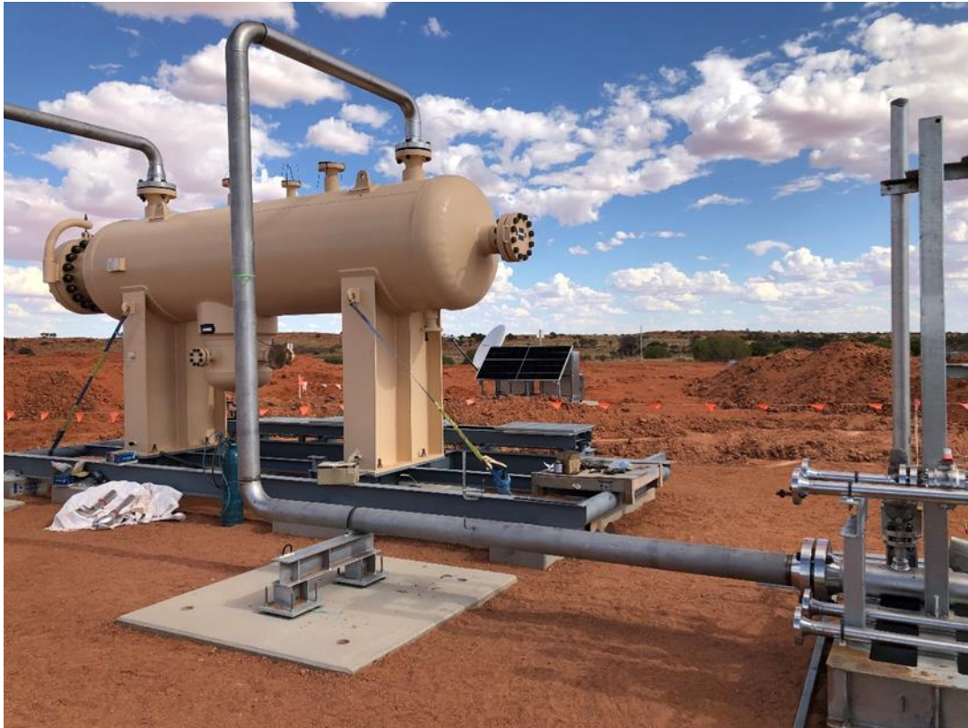
Separator installed at the Vali metering lease
