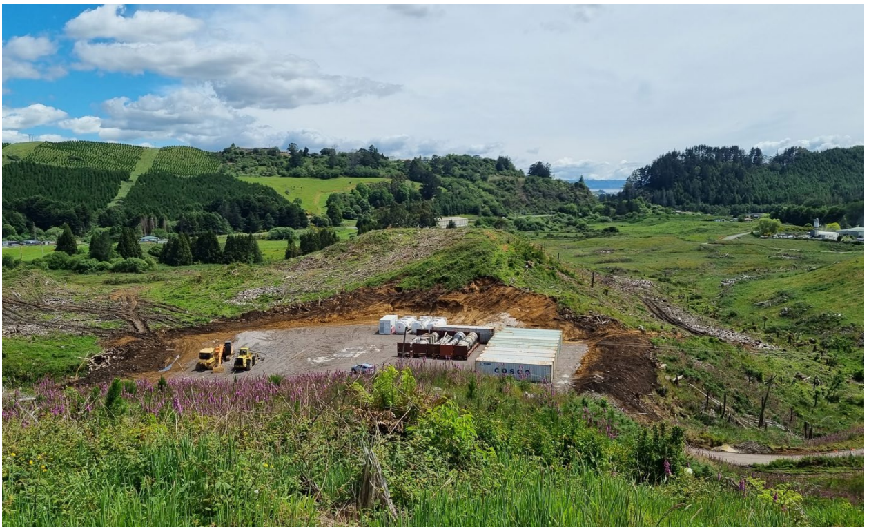
Figure 1. Plant in containers awaiting preparation for assembly and siteworks underway at the new Rotorua site
