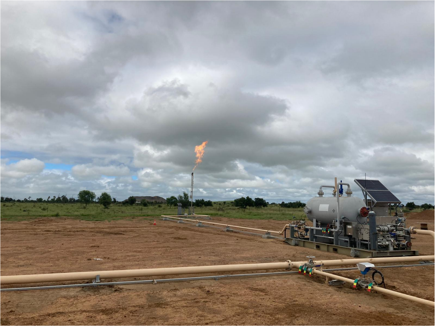
Figure 1: Gas flare during commissioning at Sapphire Pilot: Source: Blue Energy
