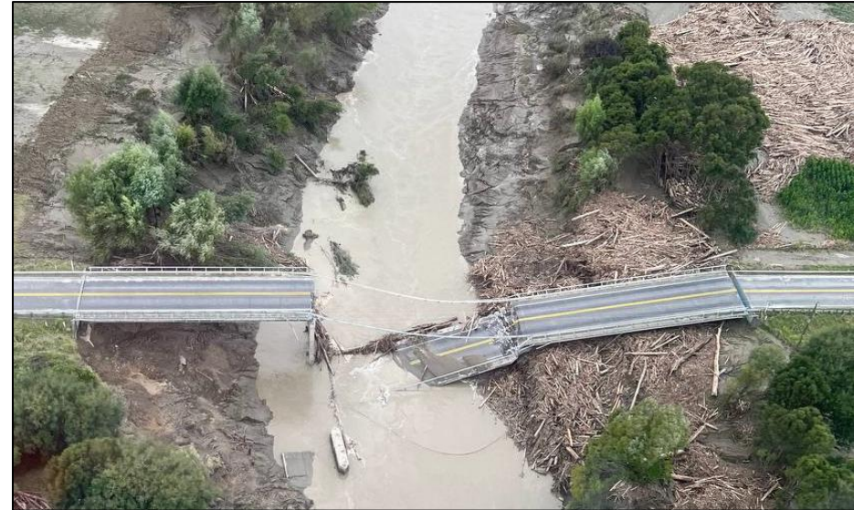
Damage to the regional fibre route on the bridge crossing the Hikuwai River, north of Gisborne, required 800 metres of overlaid fibre.
