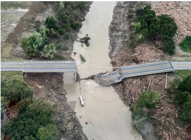
Damage to the regional fibre route on the bridge crossing the Hikuwai River, north of Gisborne, required 800 metres of fibre to be overlaid.
