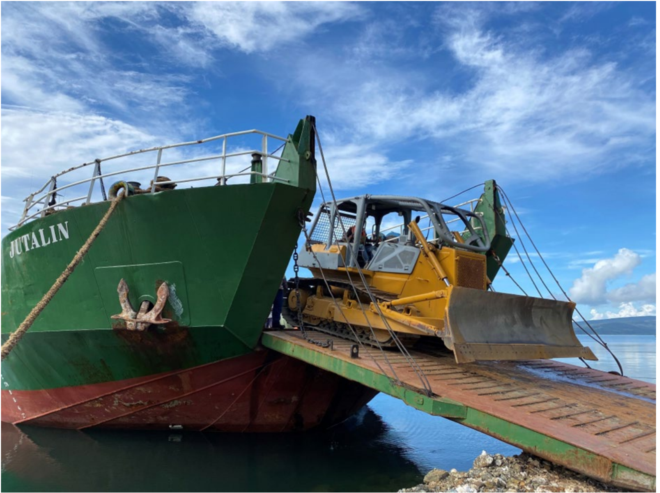
Photo 3: Local contractor equipment arriving on site for preliminary access earthworks and haul road construction
