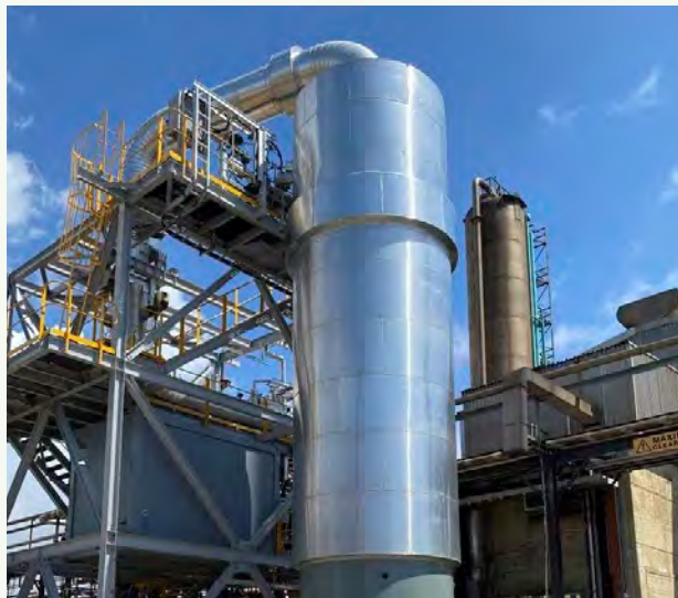
Abatement installation at Orica's Kooragang Island nitric acid plant.
