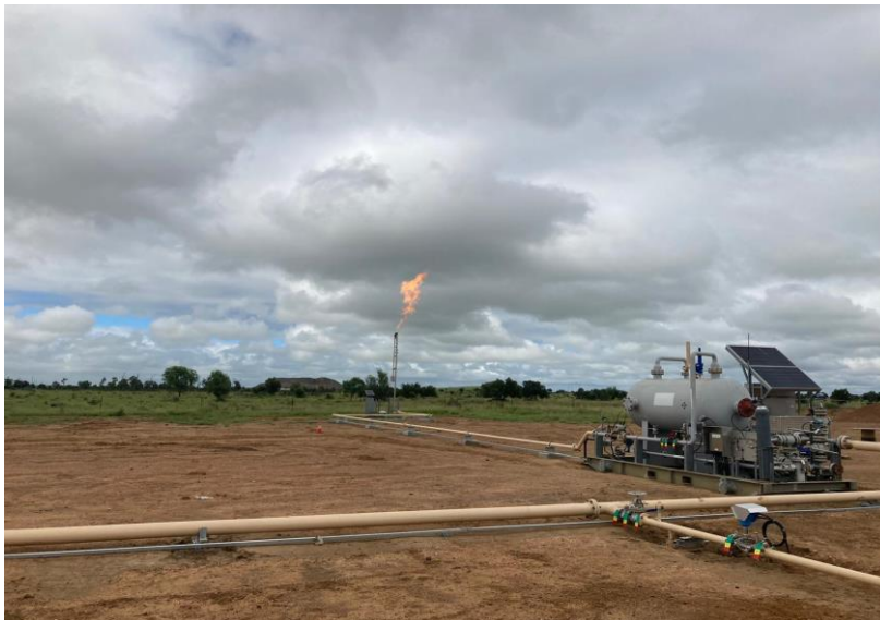
Figure 1: Gas flare during commissioning at Sapphire Pilot: Source: Blue Energy
