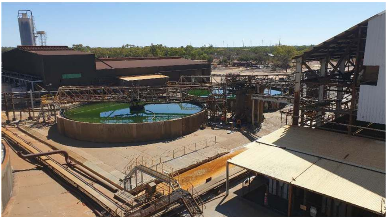
Photo 5 - Lead & Zinc Concentrates Thickeners
