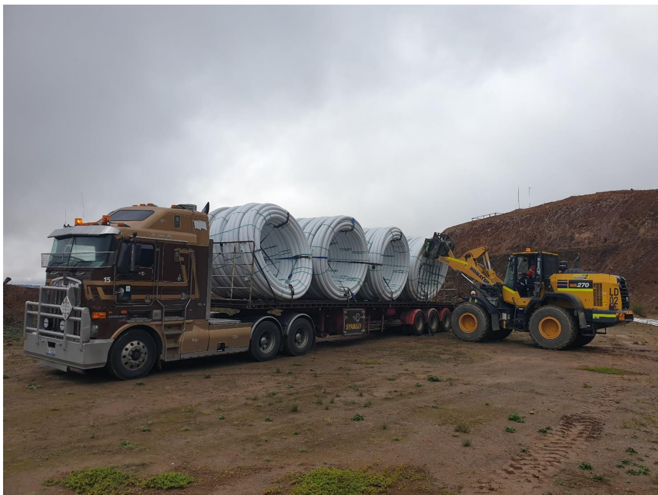
Figure 2 Unloading pit dewatering pipe
