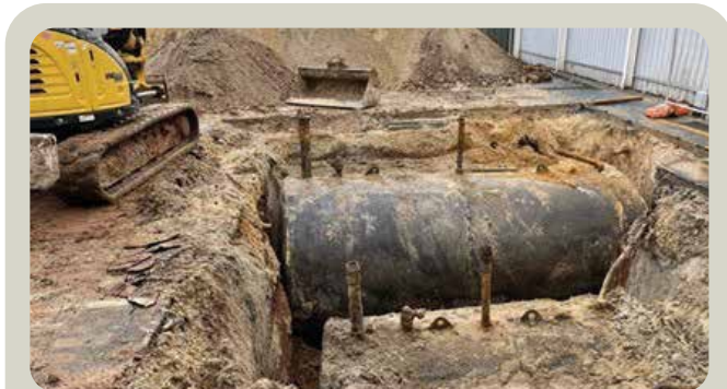
Underground Petroleum Storage System (UPSS) – One of the 37 UPSSs decommissioned, handed back or divested under our program of works to mitigate safety and environmental risks associated with UPSS.
