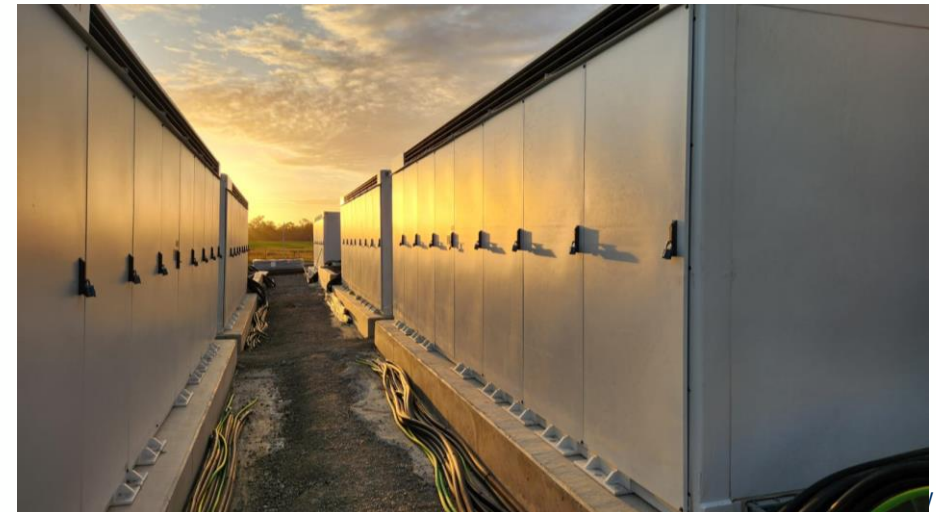
Figure 2: Tesla Megapacks at BBP Project
