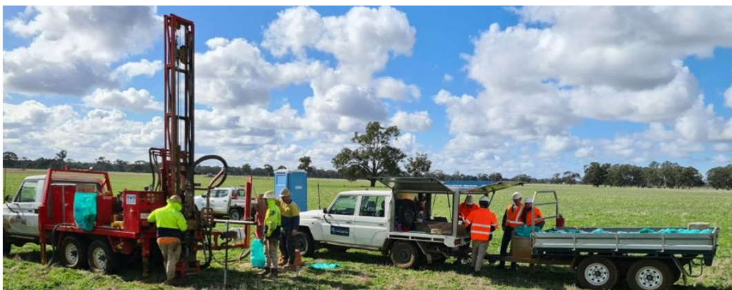
Image 1: Drilling being conducted in open paddocks of private landholdings within the Frances Exploration Target Area
